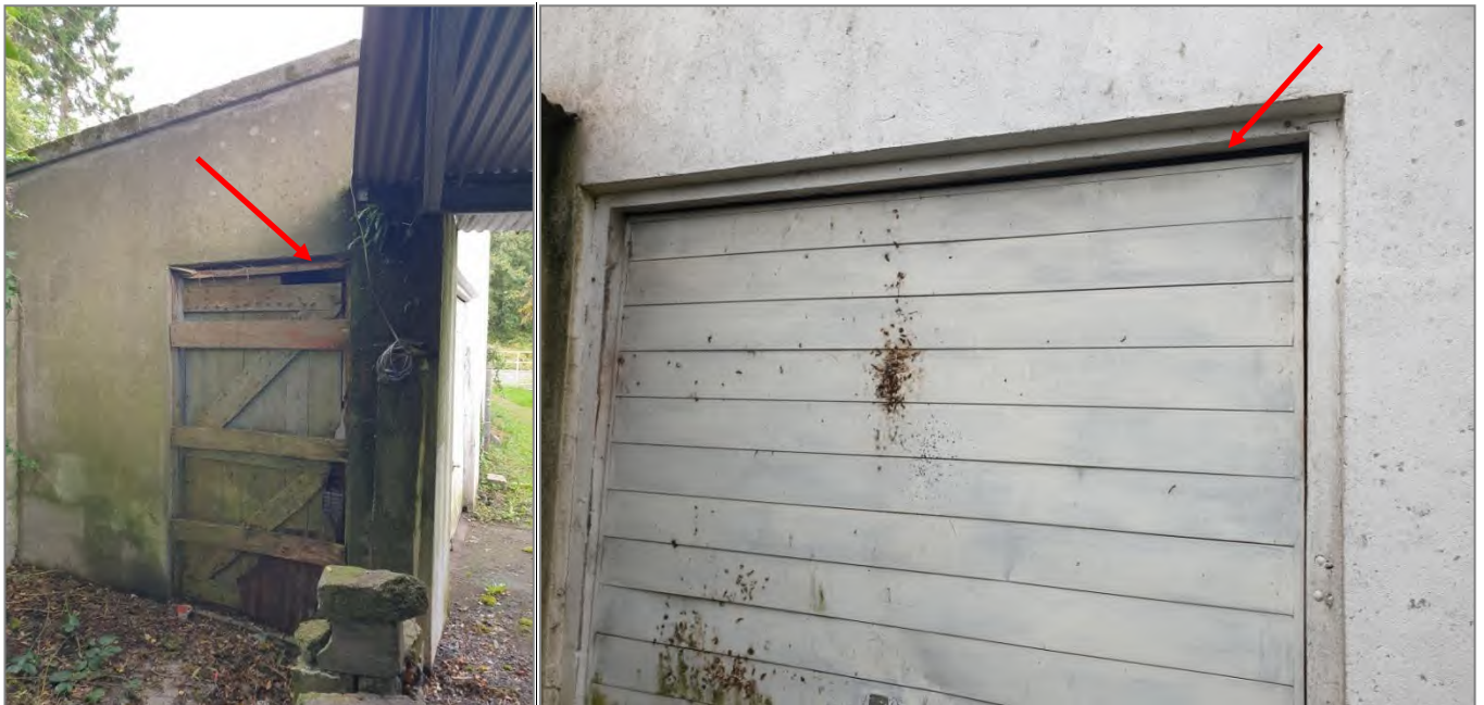
Plate 6. Potential access points for bats into sheds at cottage through gaps at the tops of doors (indicated by red arrows).
