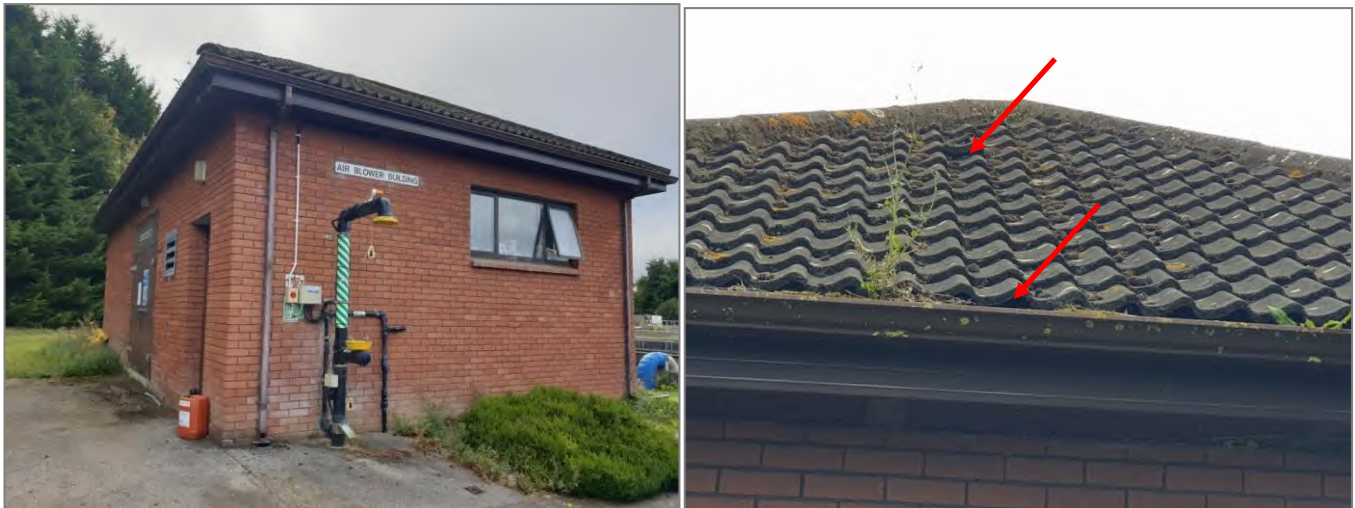
Plate 10. No bat signs but access points underneath roof tiles at Air Blower Building
